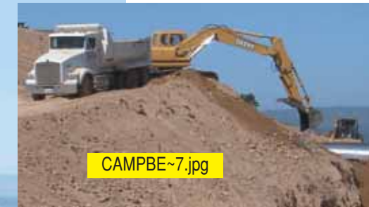
A 160LC Excavator and 700H Dozer were the main material movers during the mountain make-over.
